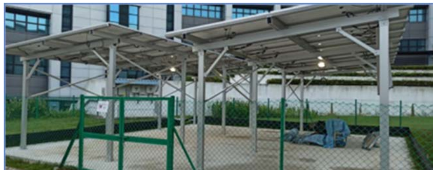
Figure 1: 16kWp Solar PV system across Plot A (L) and Plot B (R)
